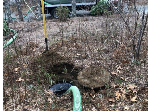
Septic Tank being pumped out
