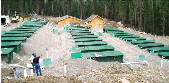
Advanced treatment units
